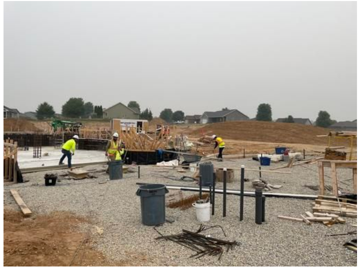
Preparing Lazy River floor Taken on Jun 28, 2023, 7:16 AM CDT Added on Jun 28, 2023, 8:59 AM CDT Added by andrew gordon
