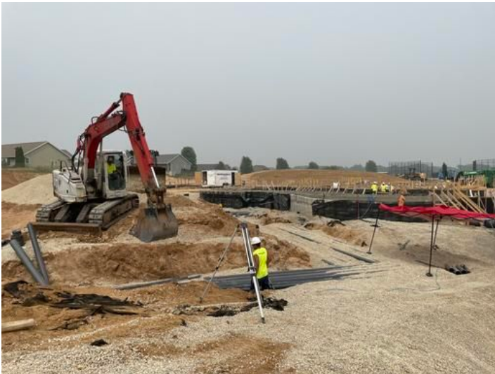
Underground pool Plumbing
