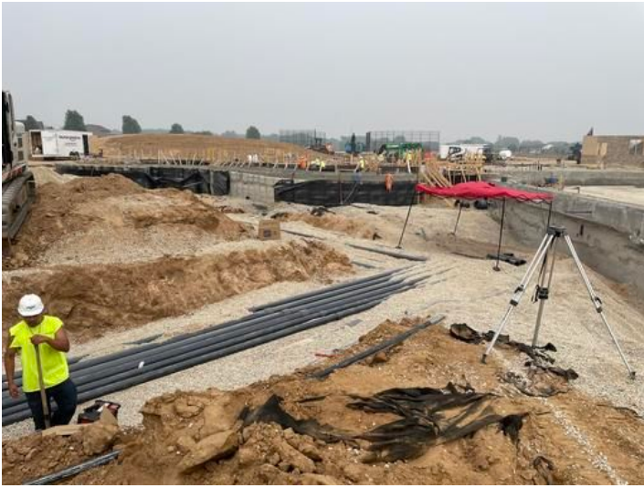
Installation of underground pool plumbing Taken on Jun 28, 2023, 3:09 PM CDT Added on Jun 28, 2023, 4:41 PM CDT Added by andrew gordon
