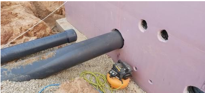
Connections of Pipe from pool to Equipment /Pump House
