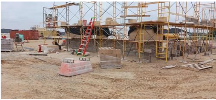
Installation of masonry on the Bath House Taken on Jun 16, 2023, 8:56 AM CDT Added on Jun 16, 2023, 10:15 AM CDT Added by andrew gordon
