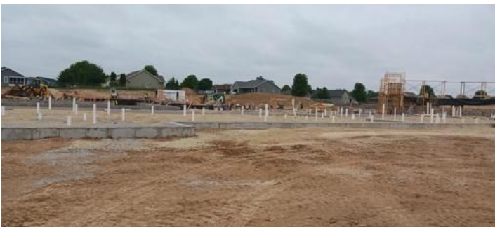
Bath House and floor plumbing Taken on Jun 16, 2023, 8:51 AM CDT Added on Jun 16, 2023, 10:27 AM CDT Added by andrew gordon
