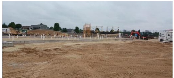
underground plumbing in the Bath House Taken on Jun 16, 2023, 8:51 AM CDT Added on Jun 16, 2023, 10:15 AM CDT Added by andrew gordon
