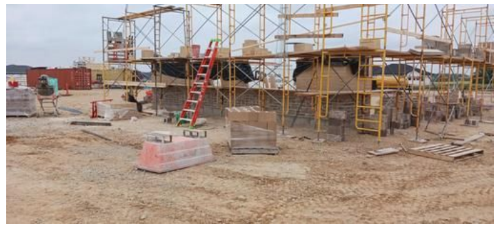
Installation of masonry on the Bath House Taken on Jun 16, 2023, 8:56 AM CDT Added on Jun 16, 2023, 10:28 AM CDT Added by andrew gordon
