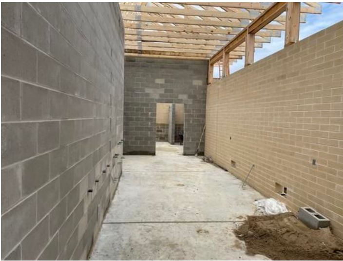
Installation of masonry walls at Bath House. Added on Sep 22, 2023, 9:36 AM CDT Added by andrew gordon
