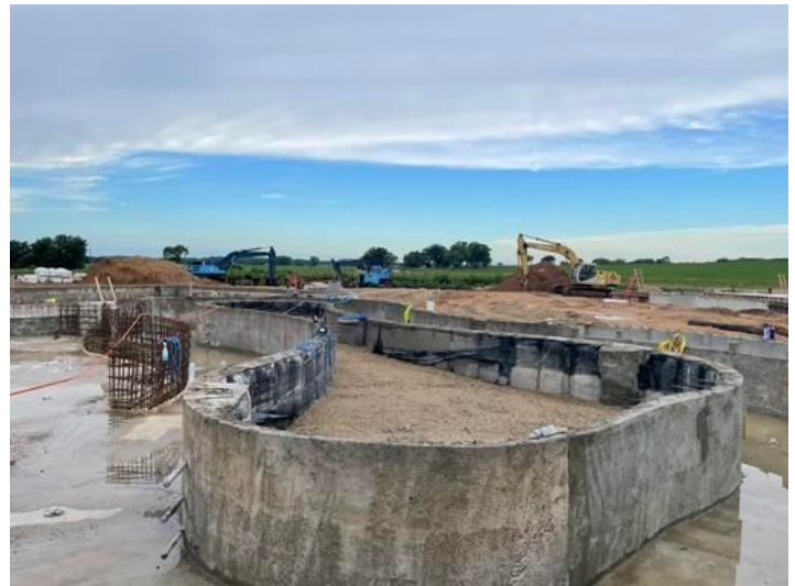
Backfill of Lazy River Pool. Taken on Jul 28, 2023, 7:06 AM CDT Added on Jul 28, 2023, 12:38 PM CDT Added by andrew gordon
