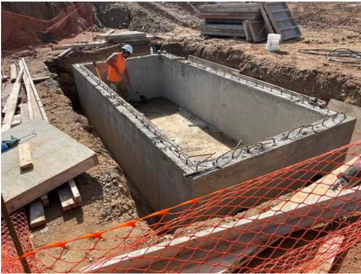
Slide surge tank Taken on Jul 28, 2023, 9:34 AM CDT Added on Jul 28, 2023, 1:05 PM CDT Added by andrew gordon
