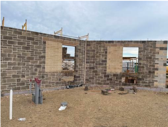
completion of masonry walls Taken on Jul 28, 2023, 7:03 AM CDT Added on Jul 28, 2023, 9:04 AM CDT Added by andrew gordon
