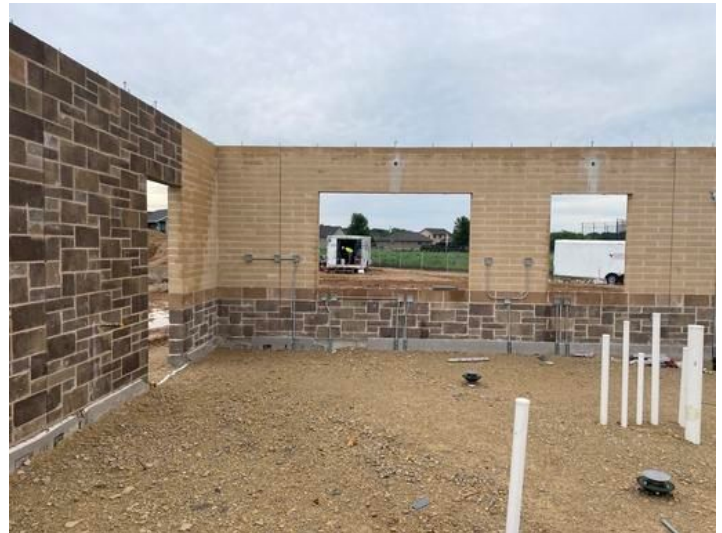
Completion of Electrical on CMU walls Taken on Jul 28, 2023, 7:03 AM CDT Added on Jul 28, 2023, 9:04 AM CDT Added by andrew gordon
