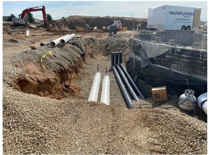
Ongoing installation of underground water slide piping Taken on Jul 28, 2023, 9:33 AM CDT Added on Jul 28, 2023, 12:39 PM CDT Added by andrew gordon
