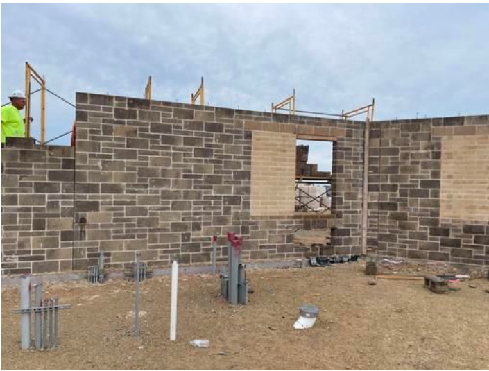
Completion of exterior Masonry walls Taken on Jul 28, 2023, 7:03 AM CDT Added on Jul 28, 2023, 9:04 AM CDT Added by andrew gordon
