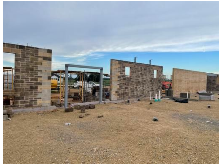
Installation of Entry steel Taken on Jul 28, 2023, 7:03 AM CDT Added on Jul 28, 2023, 9:04 AM CDT Added by andrew gordon
