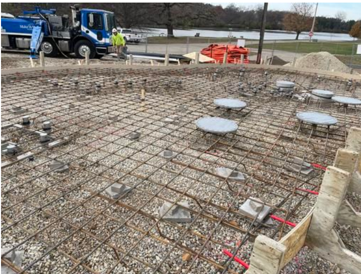
install and prep for Splash Pad concrete pour. Taken on Nov 16, 2023, 10:14 AM CST Added on Nov 16, 2023, 12:30 PM CST Added by andrew gordon
