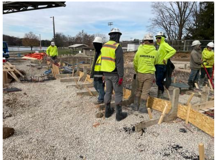
Prepare for Splash Pad concrete pour. Taken on Nov 16, 2023, 10:12 AM CST Added on Nov 16, 2023, 12:24 PM CST Added by andrew gordon
