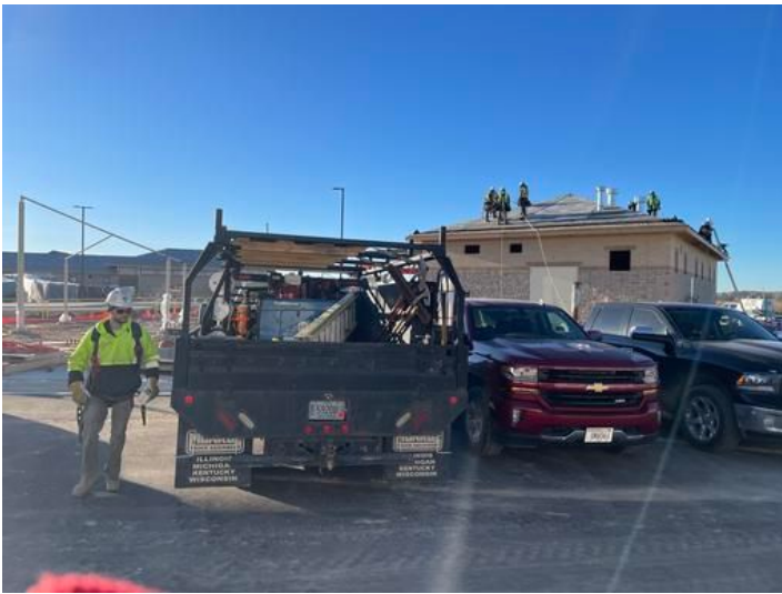
Roof installation at Pump House Taken on Nov 17, 2023, 8:27 AM CST Added on Nov 18, 2023, 9:37 AM CST Added by andrew gordon
