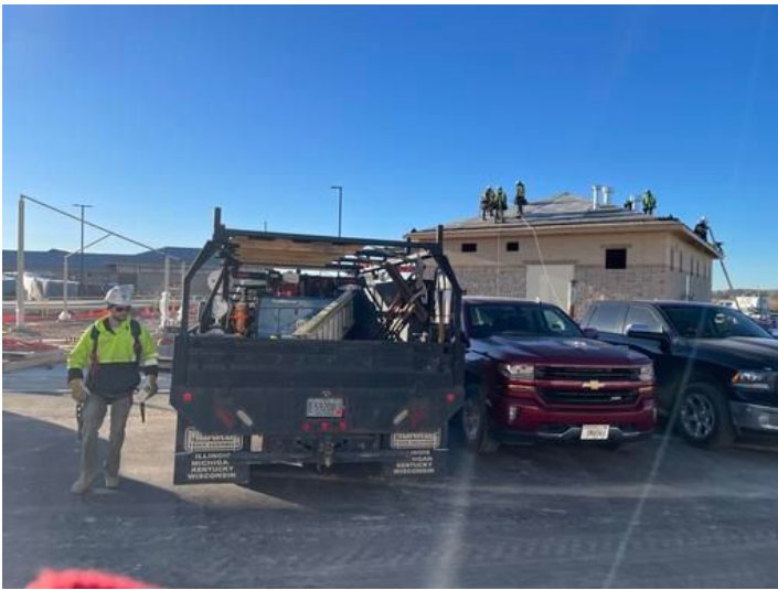
Roof installation at Pump House Taken on Nov 17, 2023, 8:27 AM CST Added on Nov 18, 2023, 9:37 AM CST Added by andrew gordon
