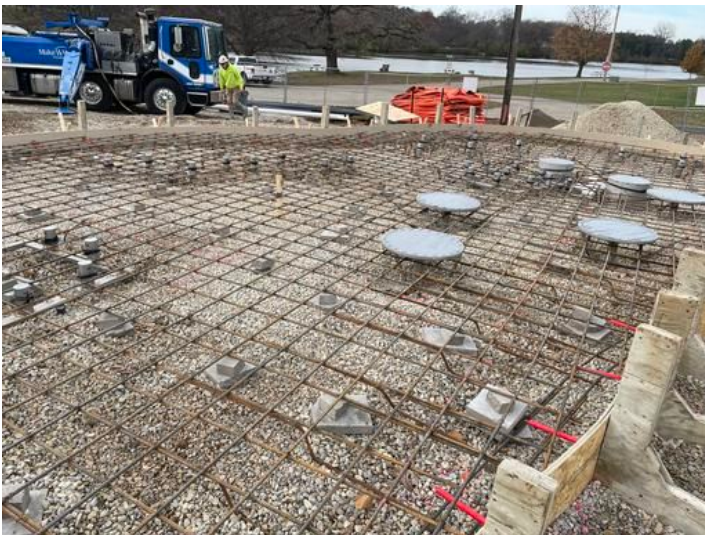
install and prep for Splash Pad concrete pour. Taken on Nov 16, 2023, 10:14 AM CST Added on Nov 16, 2023, 12:30 PM CST Added by andrew gordon
