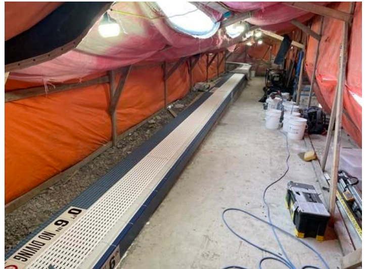
tile work for Lazy River entry. Taken on Nov 10, 2023, 9:52 AM CST Added on Nov 10, 2023, 10:33 AM CST Added by andrew gordon
