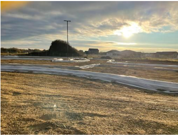
Installed Curb on South parking lot Taken on Nov 10, 2023, 7:36 AM CST Added on Nov 10, 2023, 10:40 AM CST Added by andrew gordon
