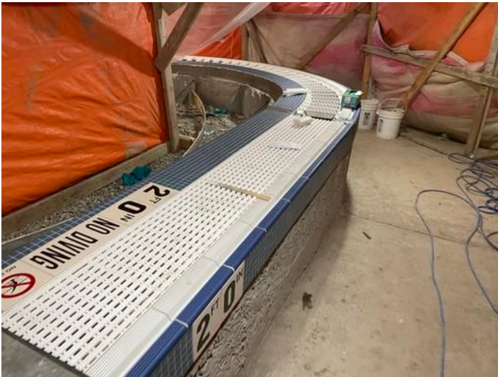
tile work for Lazy River entry Taken on Nov 10, 2023, 9:53 AM CST Added on Nov 10, 2023, 10:37 AM CST Added by andrew gordon
