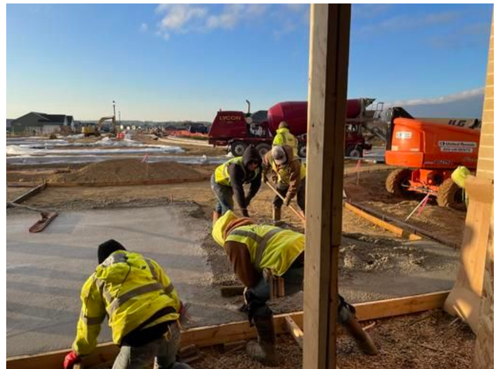
installation of front Bath House entry walkway. Taken on Nov 10, 2023, 7:30 AM CST Added on Nov 10, 2023, 10:36 AM CST Added by andrew gordon
