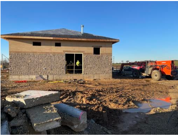
Pump House ready for grading. Taken on Nov 9, 2023, 7:49 AM CST Added on Nov 9, 2023, 8:56 AM CST Added by andrew gordon
