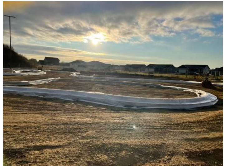
Southside Parking lot curb installed Taken on Nov 10, 2023, 7:36 AM CST Added on Nov 10, 2023, 10:40 AM CST Added by andrew gordon
