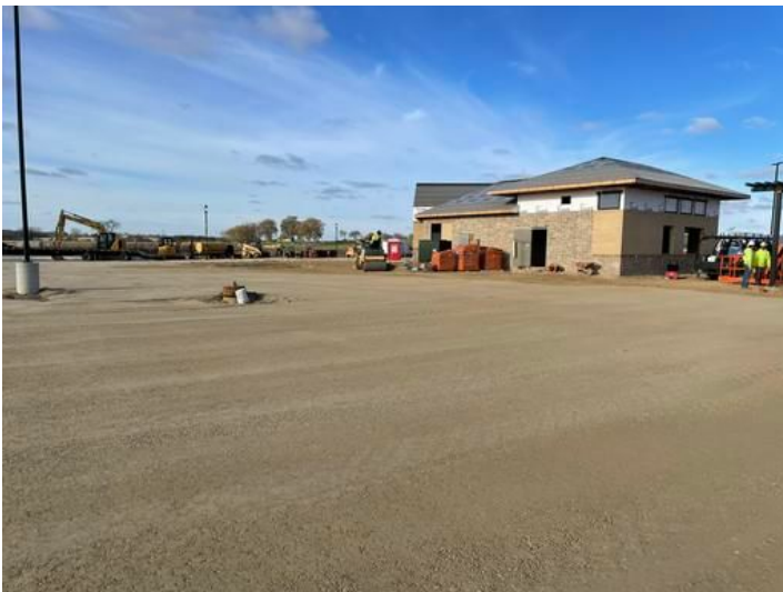
Prepare for grading of South Parking lot Taken on Nov 7, 2023, 8:42 AM CST Added on Nov 7, 2023, 2:08 PM CST Added by andrew gordon
