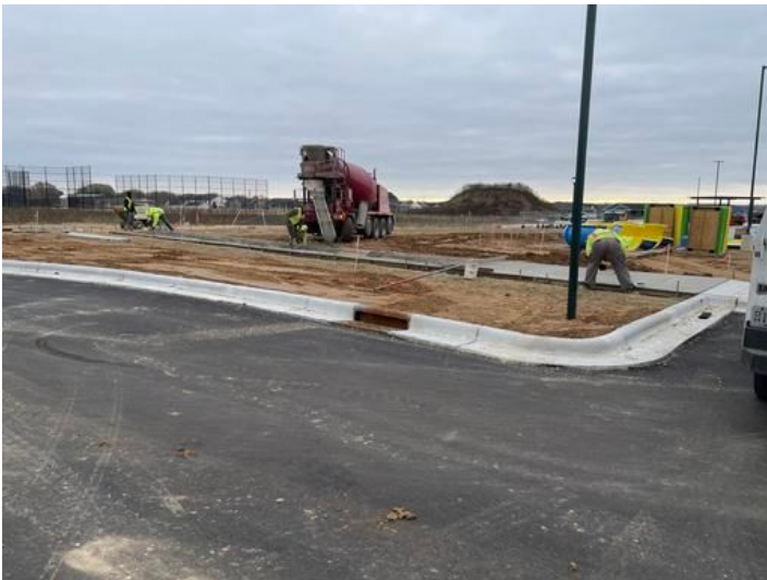
North sidewalk installation Taken on Nov 10, 2023, 9:38 AM CST Added on Nov 10, 2023, 10:36 AM CST Added by andrew gordon
