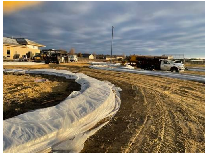
Installation of Curb on driveway. Taken on Nov 10, 2023, 7:36 AM CST Added on Nov 10, 2023, 10:39 AM CST Added by andrew gordon
