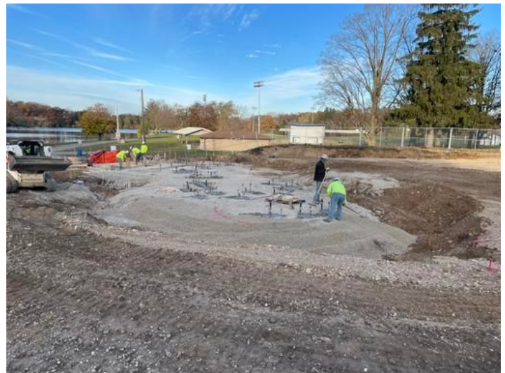
Installing underground for Splash Pad Taken on Nov 7, 2023, 7:52 AM CST Added on Nov 7, 2023, 7:54 AM CST Added by andrew gordon
