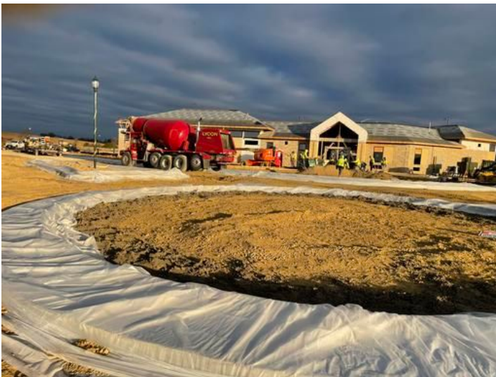
Bath House entry walkway being installed. Taken on Nov 10, 2023, 7:36 AM CST Added on Nov 10, 2023, 10:38 AM CST Added by andrew gordon
