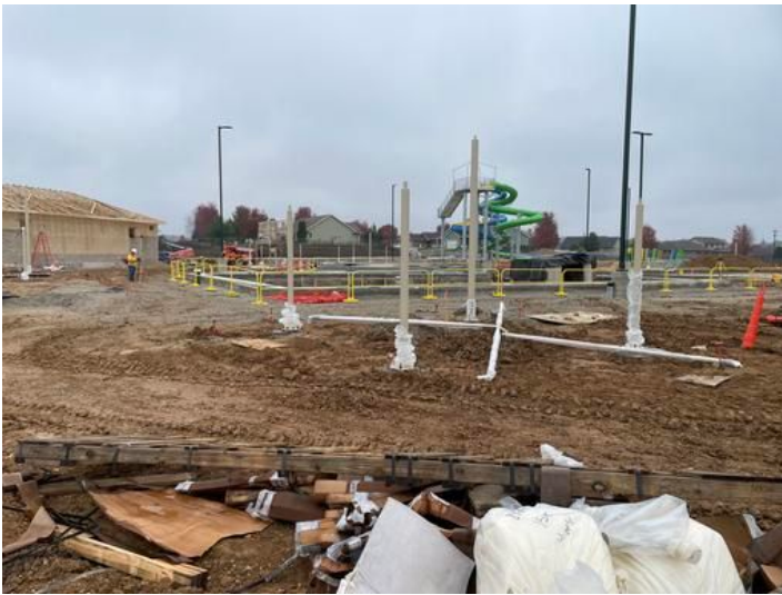
Insatallation of Sunshades Taken on Oct 25, 2023, 12:06 PM CDT Added on Oct 26, 2023, 7:55 AM CDT Added by andrew gordon
