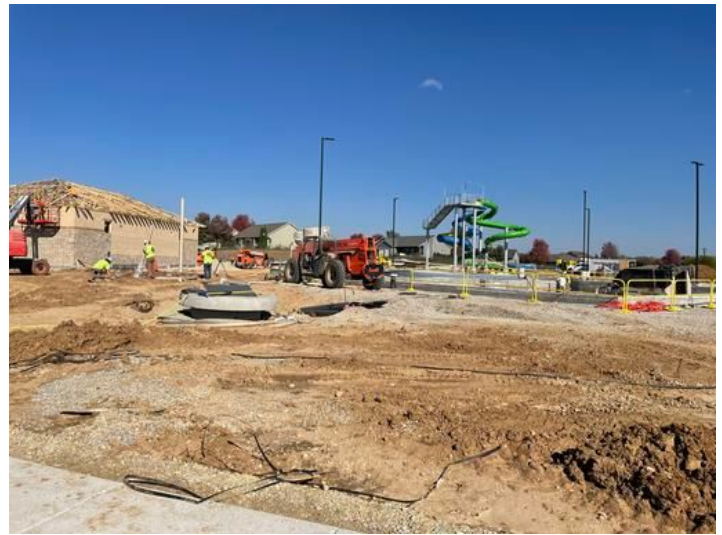
Installation Of Trusses and Sunshade. Taken on Oct 24, 2023, 1:35 PM CDT Added on Oct 24, 2023, 2:26 PM CDT Added by andrew gordon
