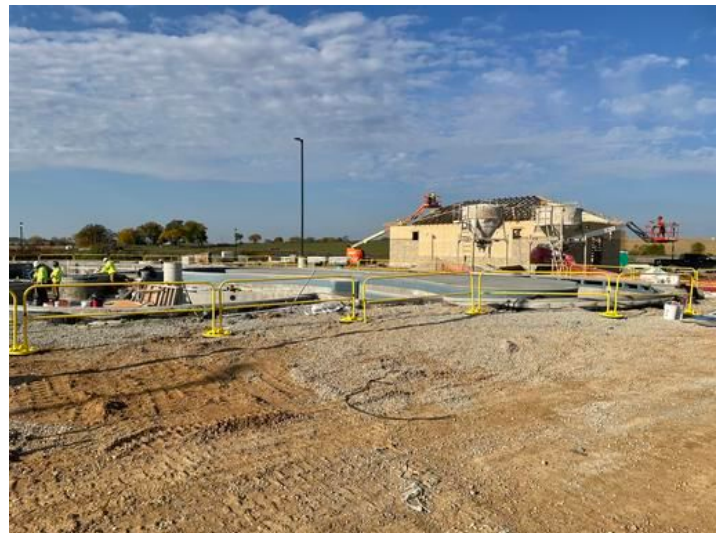
Lazy River top island poured and tile work finished. Taken on Oct 24, 2023, 10:00 AM CDT Added on Oct 24, 2023, 2:26 PM CDT Added by andrew gordon
