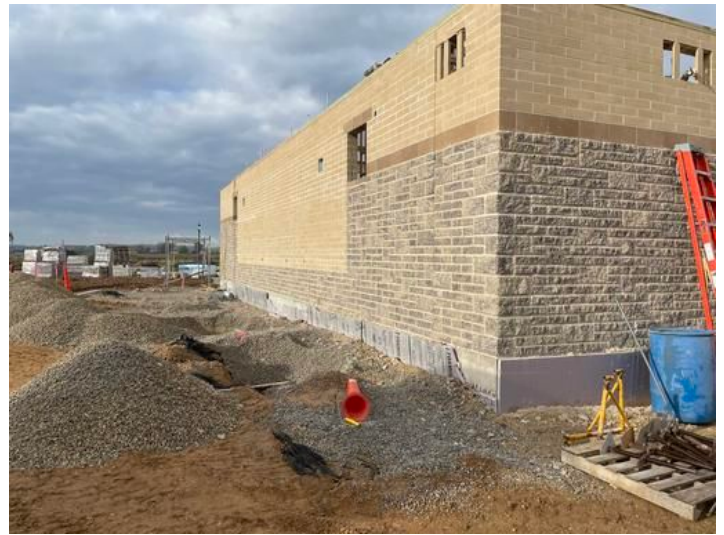
Start of trellis instalation Taken on Oct 19, 2023, 9:25 AM CDT Added on Oct 20, 2023, 8:40 AM CDT Added by andrew gordon
