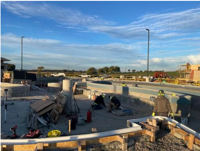
Lazy River walls Taken on Oct 18, 2023, 7:56 AM CDT Added on Oct 18, 2023, 9:34 AM CDT Added by andrew gordon
