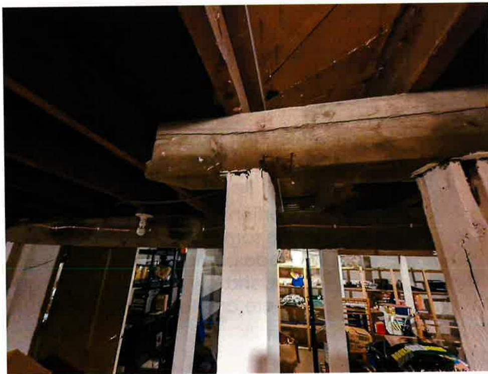
Original beam & column support. No Hanger supports. Does not meet the required 100lbs/sf floor framing requirement
