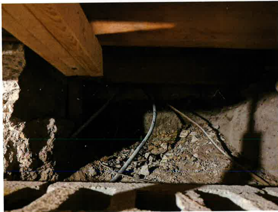
Abandoned pipes & improper supports...Slab on Grade condition is visible beyond
