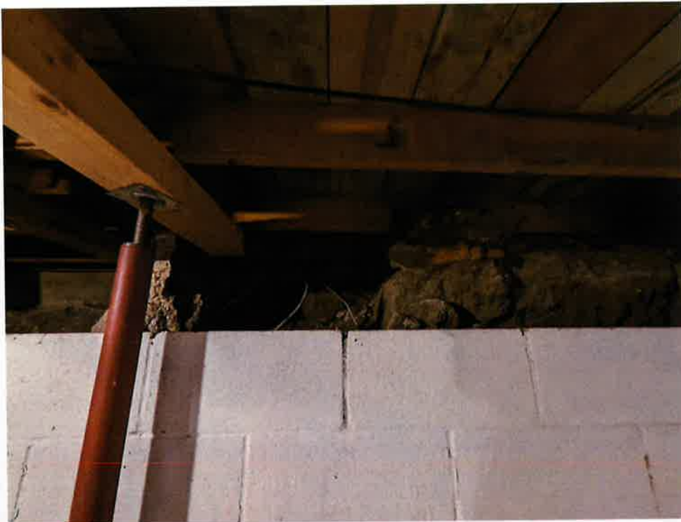
Exposed unexcavated area. Allows moisture
