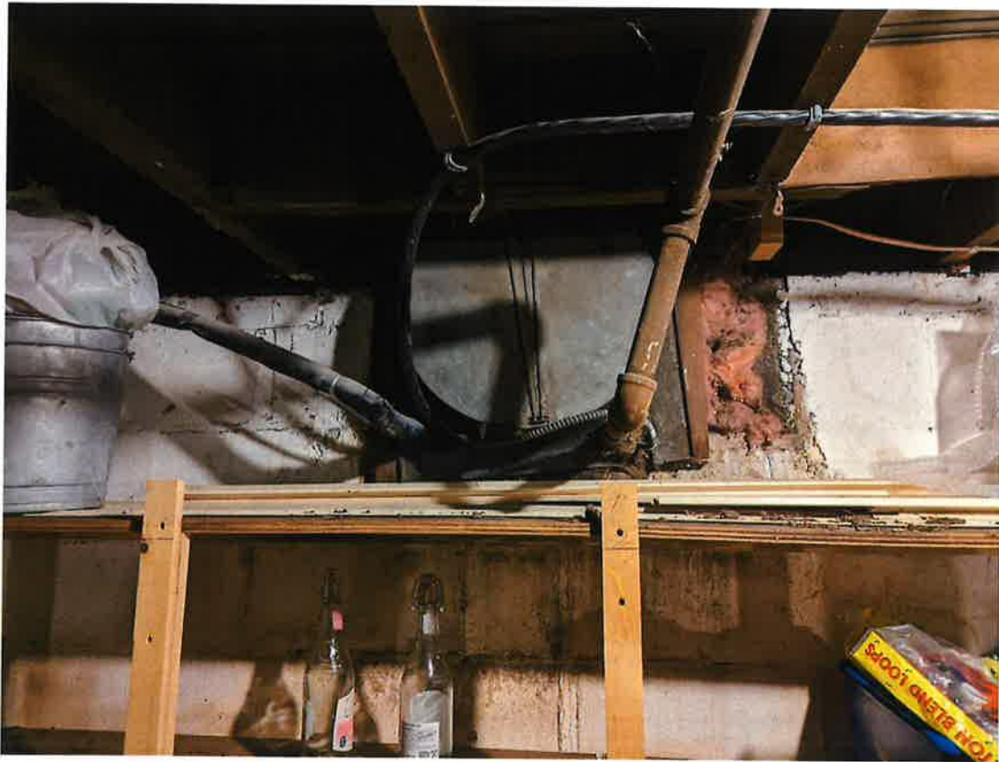
Basement mechanical chase to outside, south wall. Water stains down wall show evidence of water infiltration in the past.
