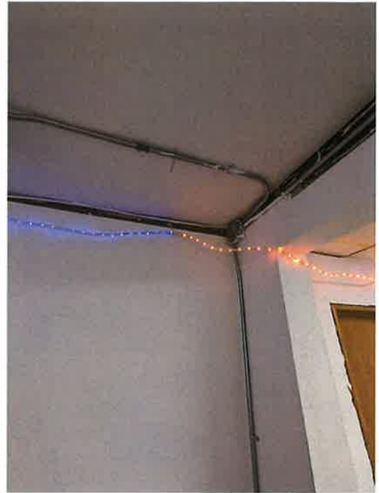
Wiring and piping in various areas are generally 'unfinished'.
