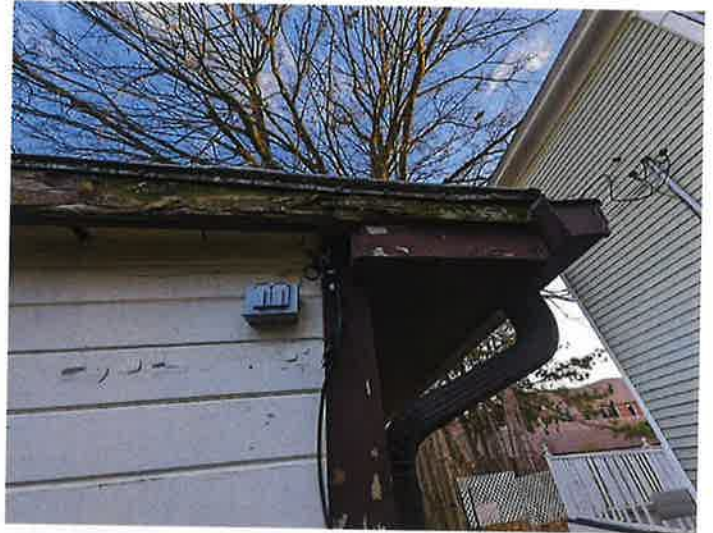
Excessive wood rot. Electrical was added to this location and it appears to have electric heat tape to avoid ice damming. This is a water infiltration area due to lack of insulation and modifying an old 'garage' into an interior space.
