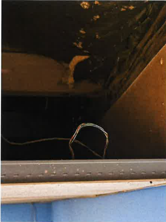
Misc. wire in ceiling. It is recommended to have an electrician inspect wiring and repair non-compliant conditions
