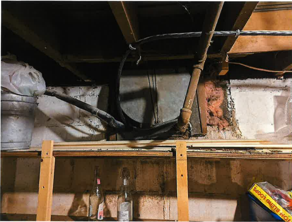
Basement mechanical chase to outside, south wall. Water stains down wall show evidence of water infiltration in the past.
