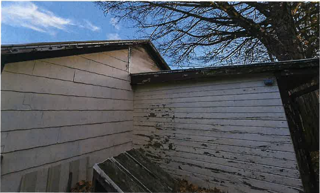
The rear of the youth center is a combination of pressed siding and wood siding. The fascia's all have significant wood rot. The exterior is poorly maintained and an eyesore to the adjacent property owners.
