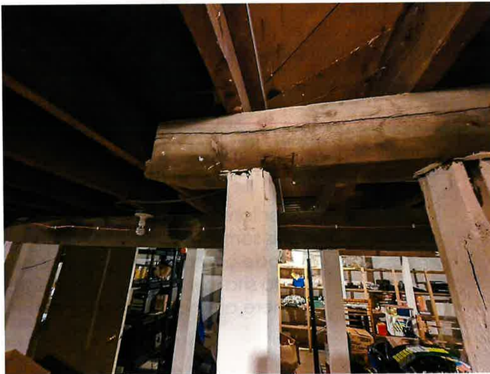
Original beam & column support. No Hanger supports. Does not meet the required 100lbs/sf floor framing requirement
