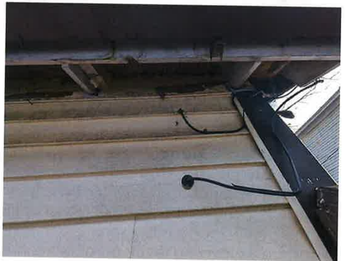
Perimeter of the building has various abandoned wires and heat tape. Electrical Services is in the rear of the building, overhead. Access is limited with the side yard of less than four feet.
