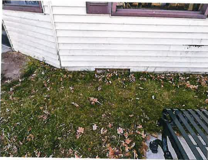
The site is flat, there is no positive grading away from the building, water susceptible building materials are deteriorating and too close to grade. 8" above grade for wood is required by code.
