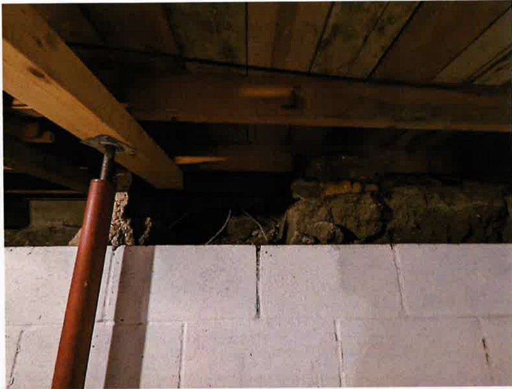
Exposed unexcavated area. Allows moisture
