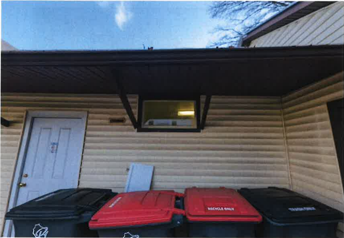
The north roof overhang is sagging. The existing bracing is not properly reinforcing the roof framing. The trash cans being located on the side yard is a visual eyesore.
