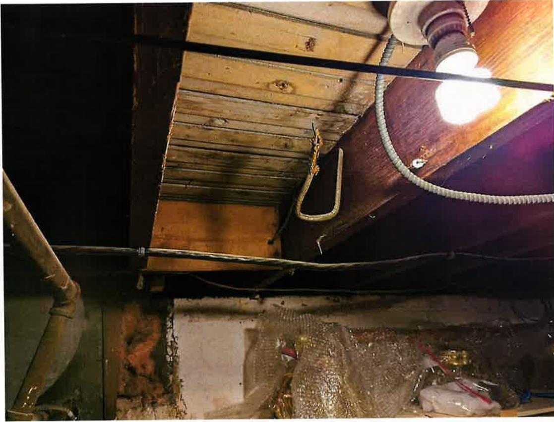
Abandoned electrical not properly terminated
