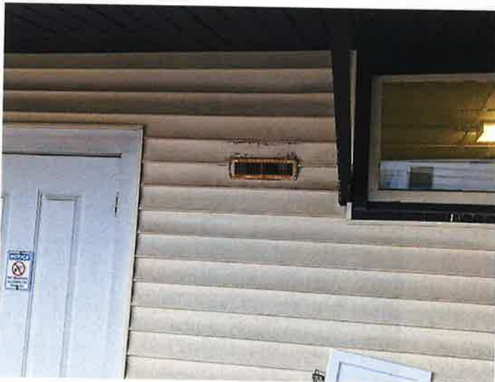
Rusted exterior exhaust vent. The building has many abandoned exterior penetrations, reflecting a concern for moisture migration through the exterior envelope and poor energy efficiency.
