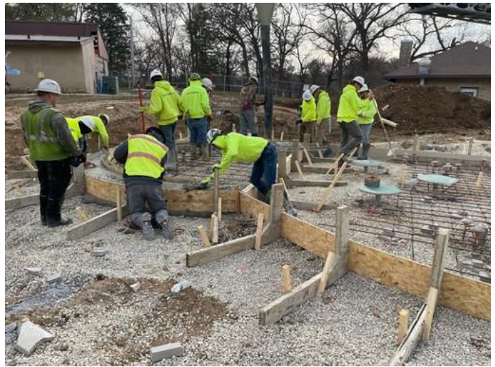
Installation of Splash Pad concrete Taken on Nov 16, 2023, 10:16 AM CST Added on Nov 16, 2023, 12:29 PM CST Added by andrew gordon
