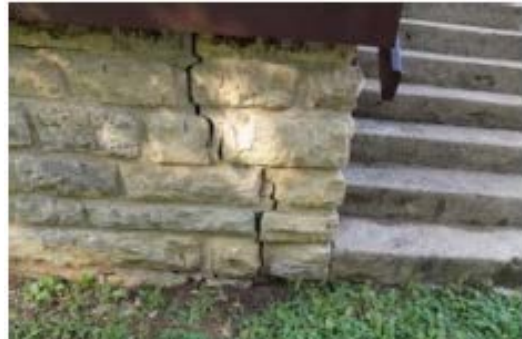
FIG. 2.6: WARMING HOUSE DETERIORATION
