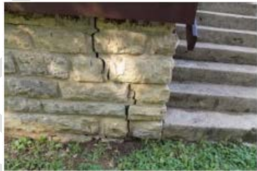
FIG. 2.6: WARMING HOUSE DETERIORATION
