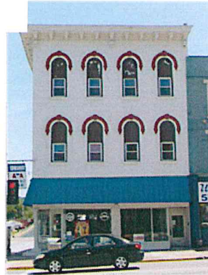
In this example, notice the replacement windows do not fit the masonry opening of the original window. Instead the new window was reduced in size dramatically changing the historic appearance of this commercial building. Source: Bob Yapp
